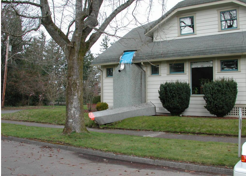
Figure 6. Typical chimney damage in the south Capital neighborhood, where many chimneys were completely destroyed.
