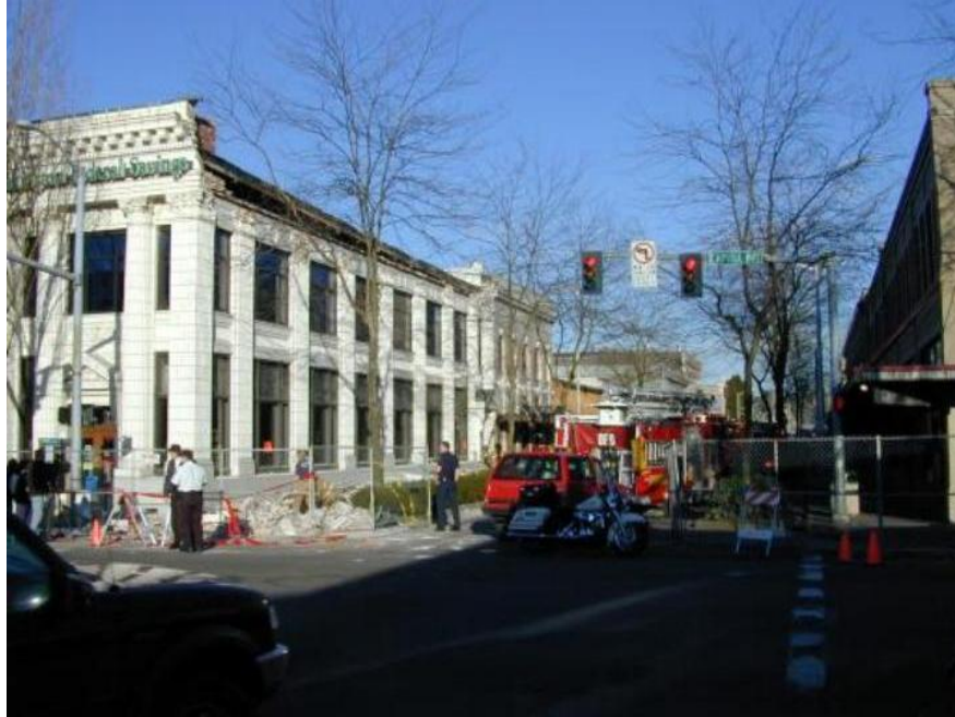
Figure 8. Parapet failure at the Washington Federal Savings Bank (an older unreinforced masonry building) in downtown Olympia, which suffered significant damage during the 2001 Nisqually earthquake .
