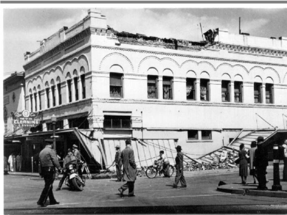
Figure 9. This unreinforced masonry building in downtown Olympia was damaged in the 1949 earthquake. Damage was extensive to this type of building in that event. This building is about one block east of the Washington Federal Savings Bank in Figure 8.
