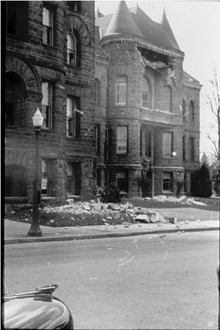
Location 1a. Damage to “old state capitol bulding” in the April 13, 1949 earthquake. Photo supplied by Jim Sims.
