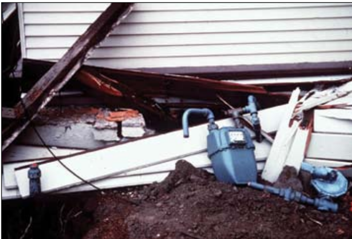
This house shifted off its foundation, breaking the utility lines and leaving it uninhabitable. Newer building codes require a house being tied to the foundation, but homeowners may need to retrofit older homes. Photo: USGS
