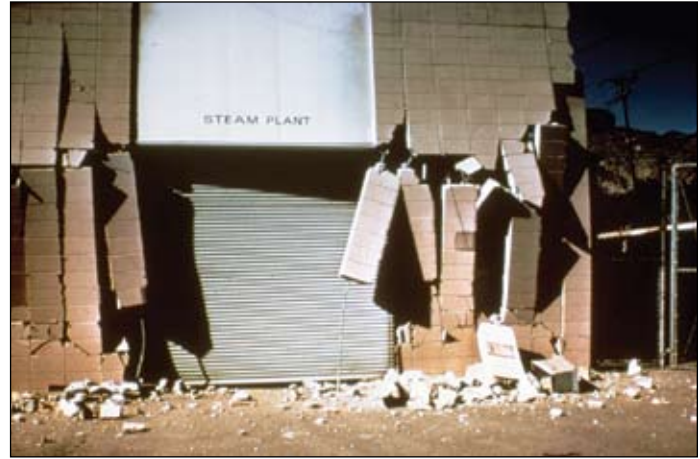
The 1971 San Fernando earthquake substantially damaged these Juvenile Hall facilities. A portion of the two-story administration building collapsed completely into the first story. Photo: E.V. Leyendecker, USGS
