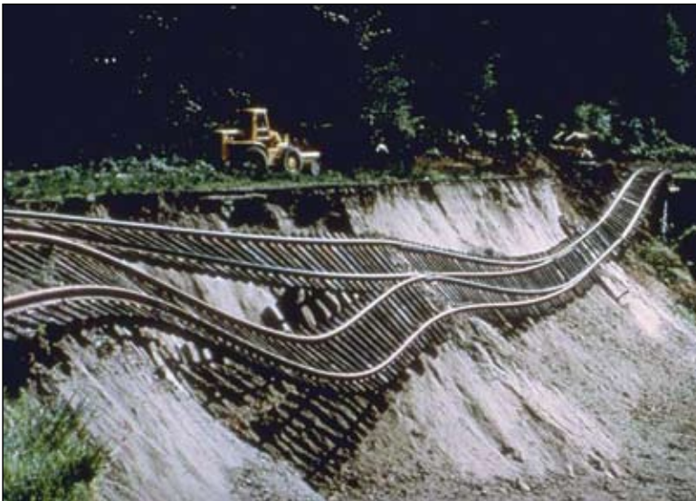
Landslides are an often-overlooked danger of earthquakes. They are particularly likely during rainy, water-soaked winter months in Cascadia. Almost 40 miles (60 kilometers) from the epicenter, this section of the Union Pacific Railway was left dangling after the hillside fill beneath it slid away in the 1965 earthquake. A sewer main also broke. Photo: University of California, Berkeley
