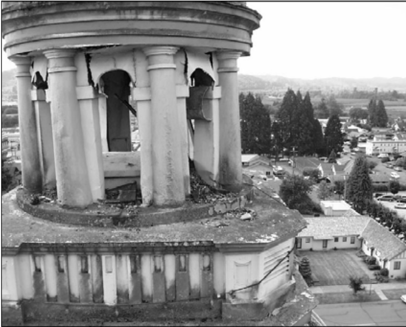
The historic Grays Harbor County Courthouse in Montesano, Washington suffered several million dollars' worth of damage in the 1999 earthquake. Photo: Grays Harbor County
