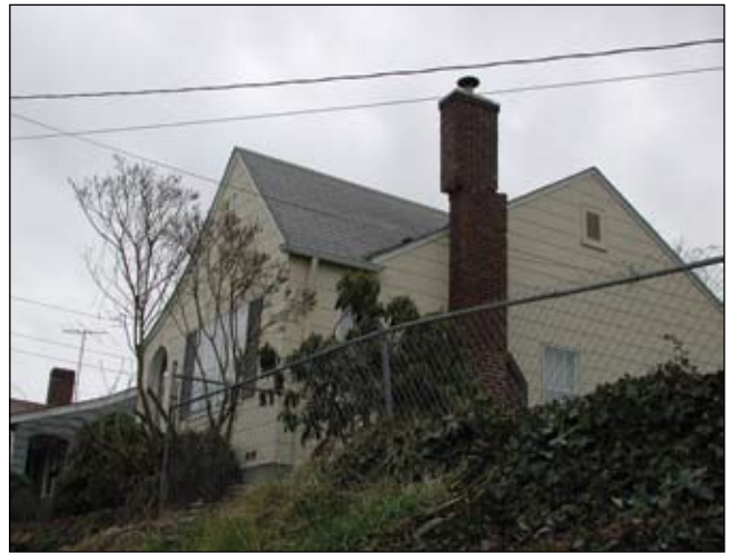
Chimney failures are a common problem for homeowners after an earthquake. The above chimney did not fall but remained a safety hazard until it was rebuilt. Photo: Michael Polenz, DGER
