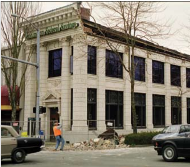
This photo of a building in Olympia after the 2001 Nisqually earthquake shows typical damage from a deep earthquake. A major source of injury is falling parapets, such as those seen above. Photo: Josh (Robert) Logan, DGER
