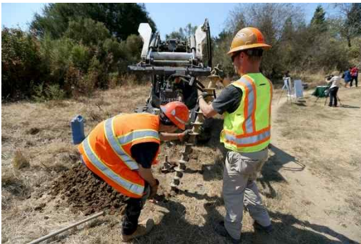
Above: Cal State East Bay graduate students drill 20-30 feet down into the ground along a trail at Lake Chabot Regional Park in Castro Valley. Photo: Anda Chu — Bay Area News Group
